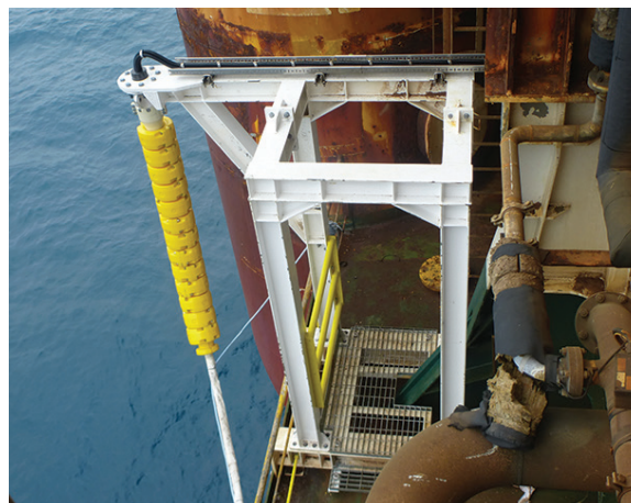
HANGING AROUND THE PORCH The anode module is suspended from this porch during normal operations.
