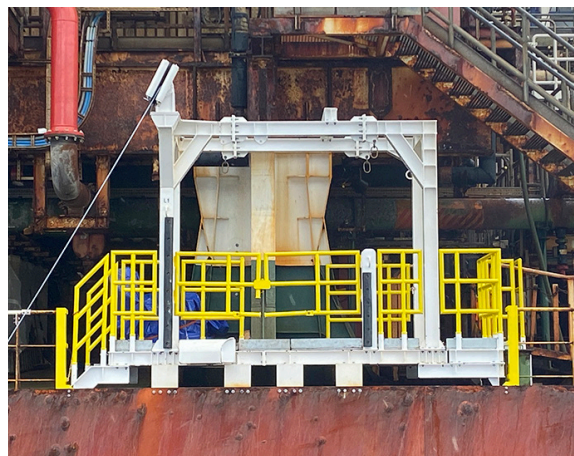
ANY PORCH IN A STORM The anode module is hoisted aboard this porch during harsh weather.
